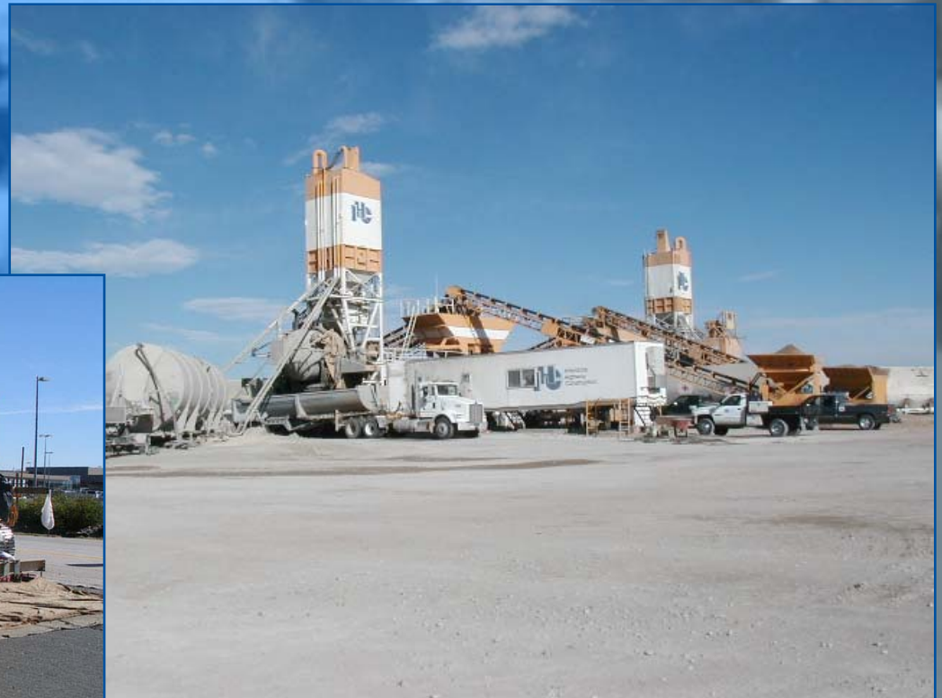
Concrete Batch Plants
